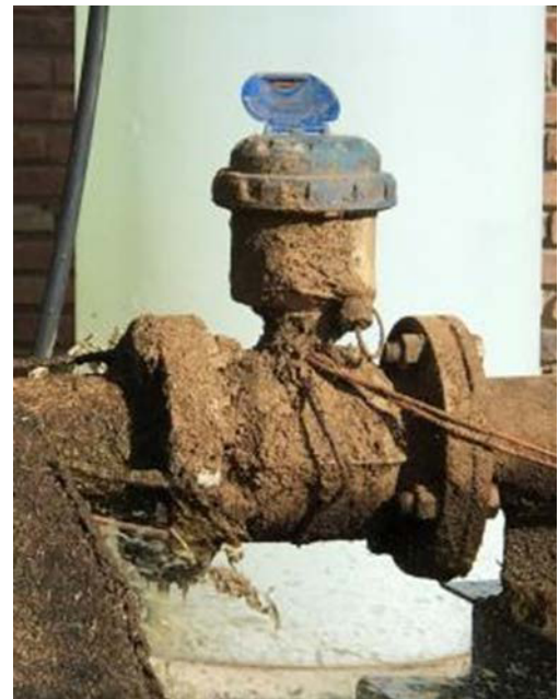
A well-used KROHNE WATERFLUX 3070 magnetic water meter in the field
