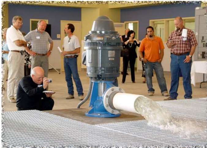
Visitors observe the flow from a 50 horsepower water pump in the ICWT laboratory. The pump sits over a 22-foot deep sump that holds 53,000 gallons of water. The pump is driven by solar energy derived from panels on the roof.
