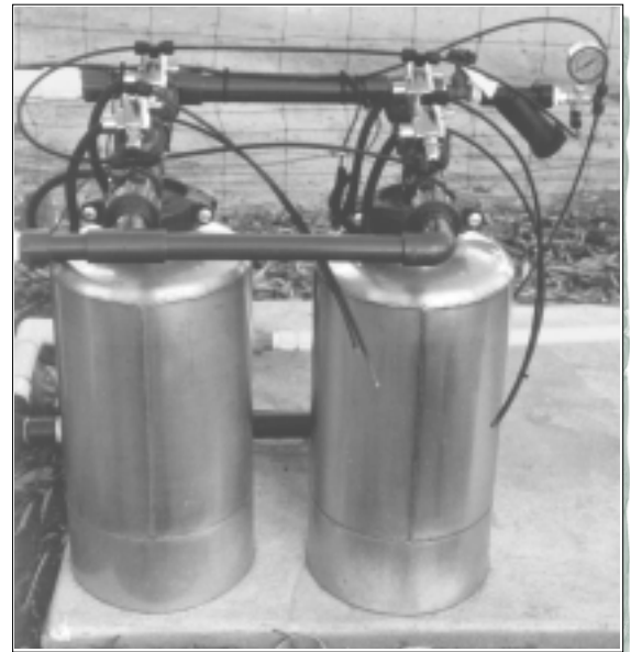
Sand media filter used in CIT study included two units: the second was used to filter water used in backflushing first unit.
